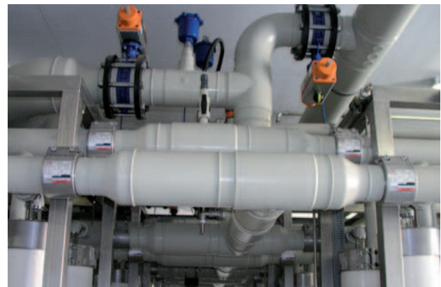
Water treatment application; connections between the racks
