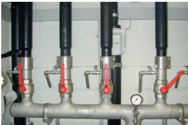
Connection of PE and stainless steel pipes, which have been installed in a well room
